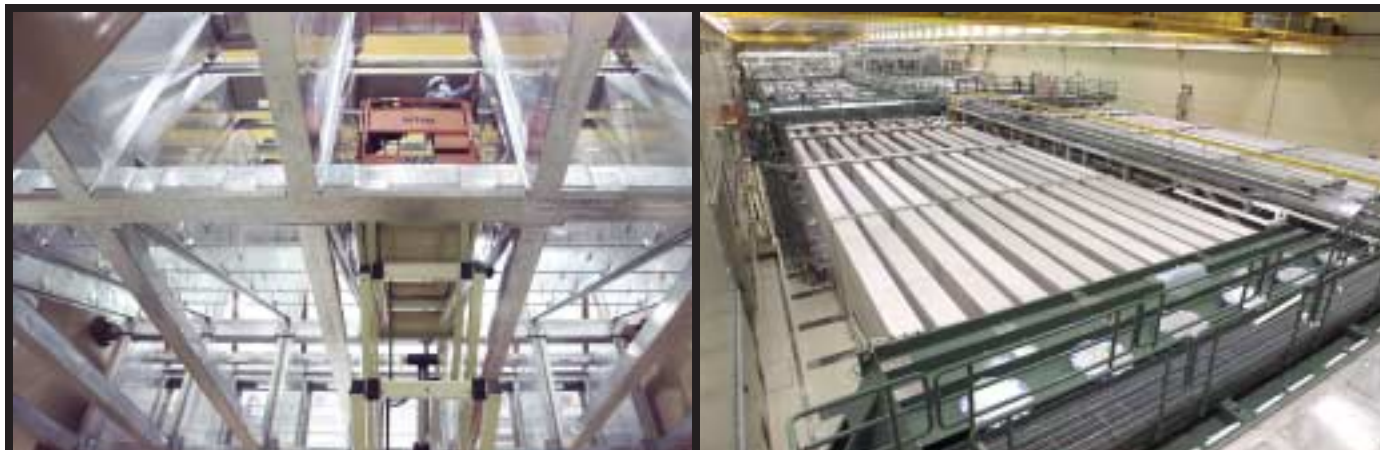
HIGH STANDARDS of cleanliness dictated that nickel-containing S30400 stainless steel be used in the target chamber of the NIF laser (left). The US$2.5-billion laser will be 200 metres long and 85 metres wide (right).
